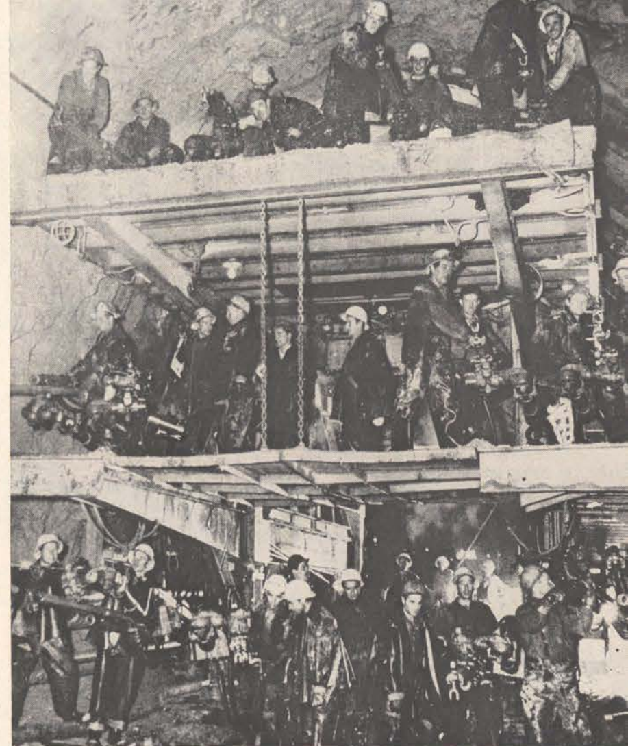
Tunnellers rig up scaffolding at the face of the Tumut 2 tailrace tunnel. The 280,000-kilowatt Tumut 2 project is the second of five hydroelectric developments on the Tumut River. The power station itself is 800 feet underground.
